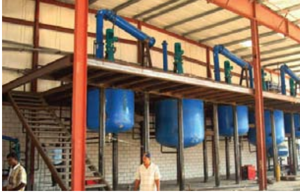
Figure 11: Resin Production Equipment (YD-FS-005)
